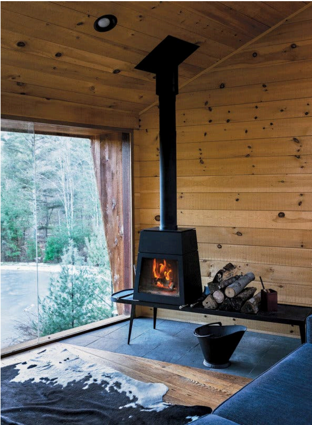
The interior designer Antony Gibbon installed a Danish steel stove from the New York-based company Wittus in the main living space; its lines echo the slope of the pine wood interior. Credit...Blaine Davis
